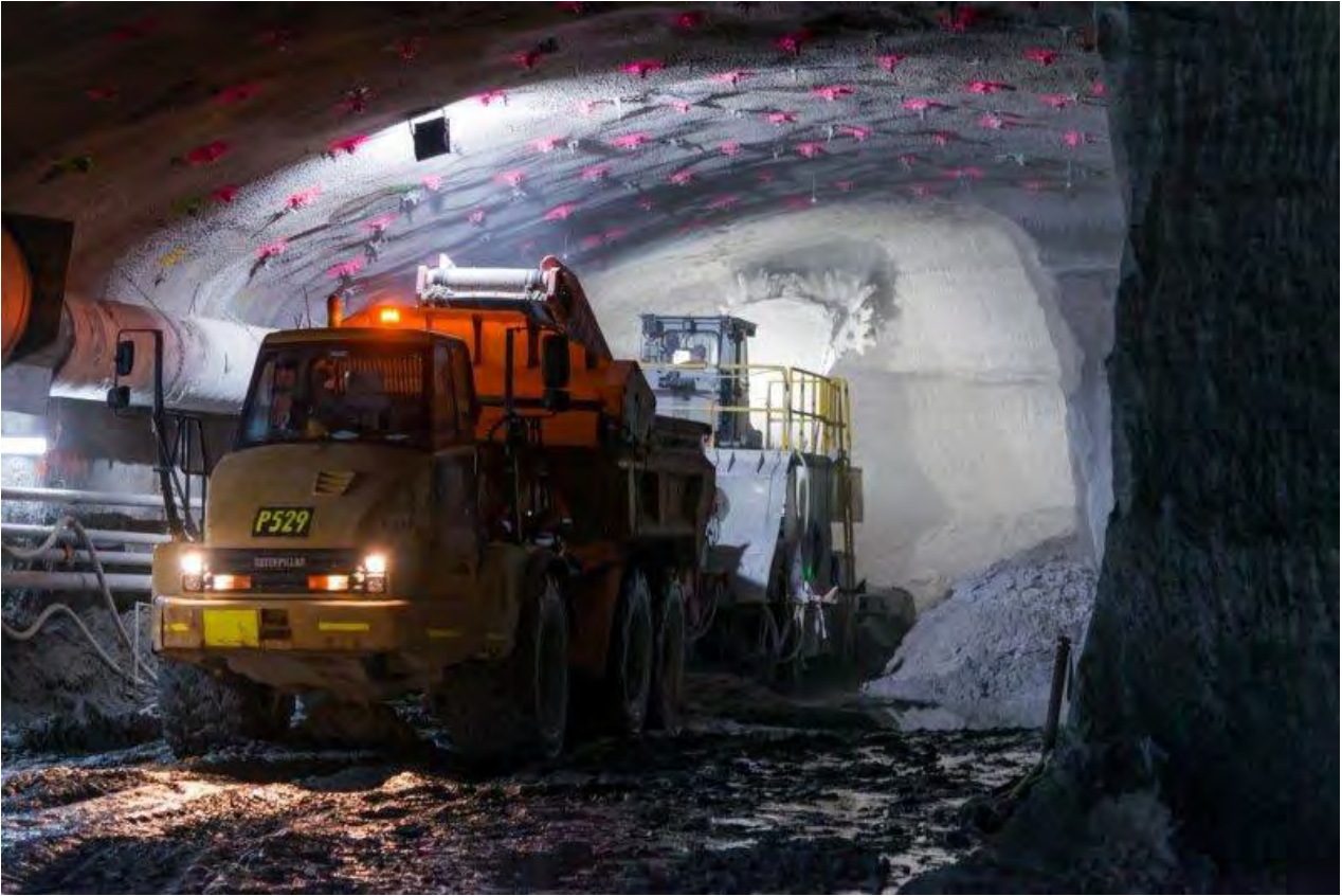
Figure 6-4 Example of a roadheader in the New M4 tunnels loading tunnel spoil into a spoil haulage truck
