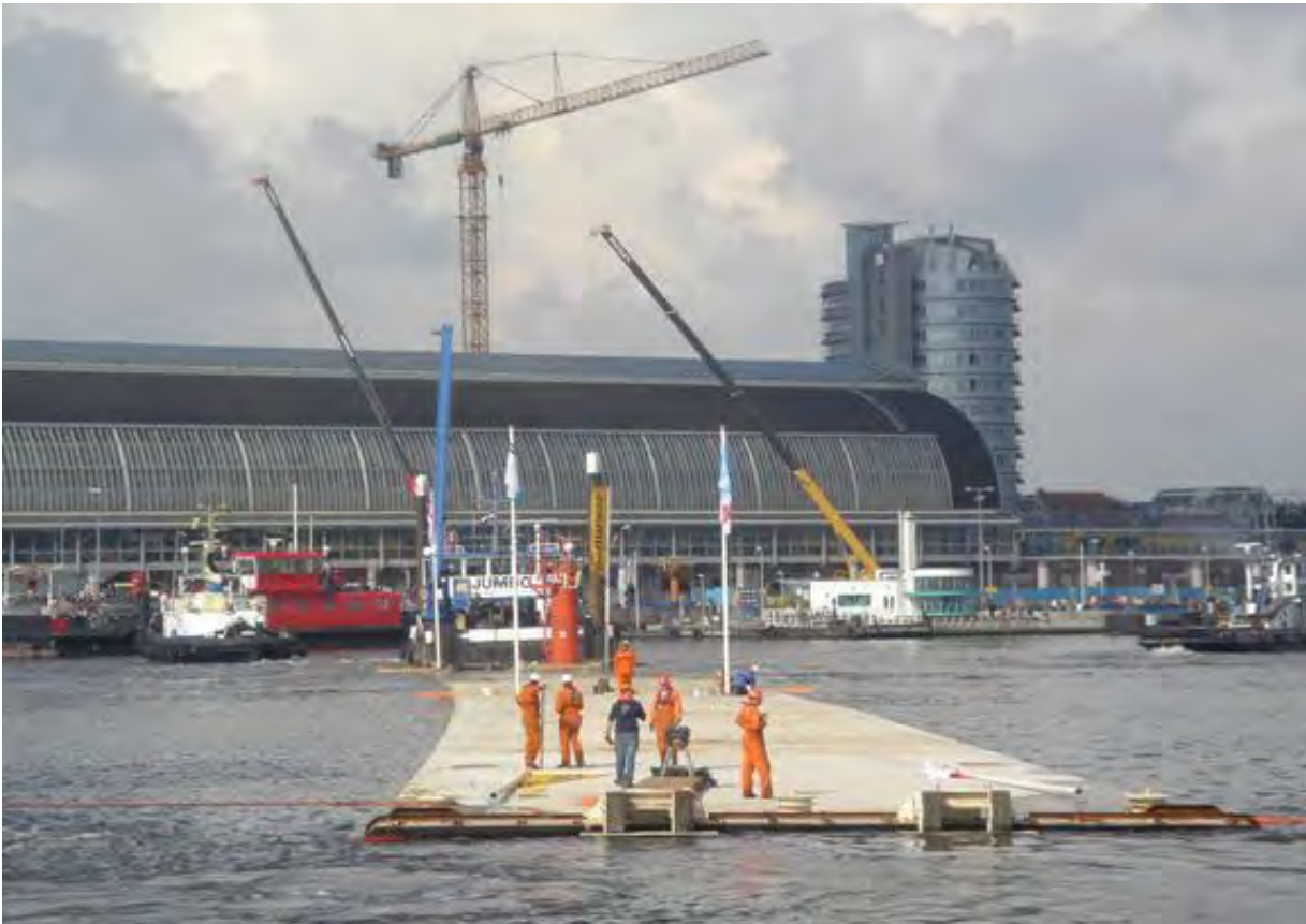
Figure 6-17 Example of completed immersed tube tunnel unit for the Amsterdam Metro moored ahead of installation (Source: ITA, n.d.)
